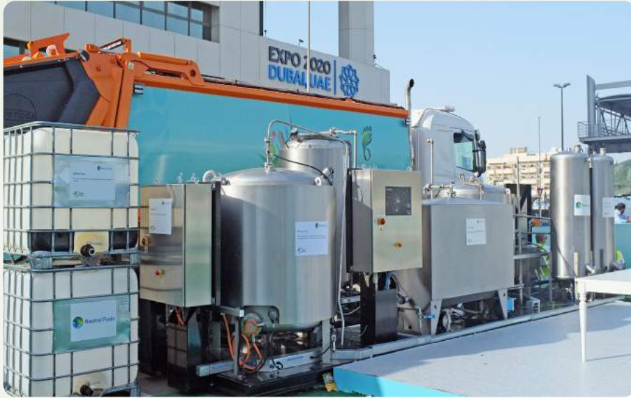
Neutral Fuels' system for producing biodiesel from used cooking oil
