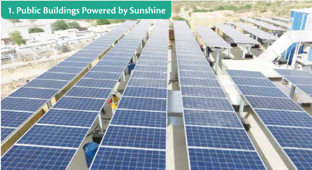
PV modules installed on the rooftop of Rashid Abdullah bin Omran Hospital
