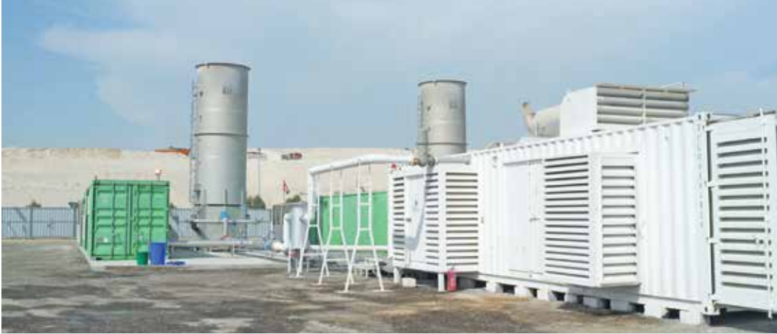
Landfill gas capture and power generation facility in the Al Qusais landfill site, Dubai
